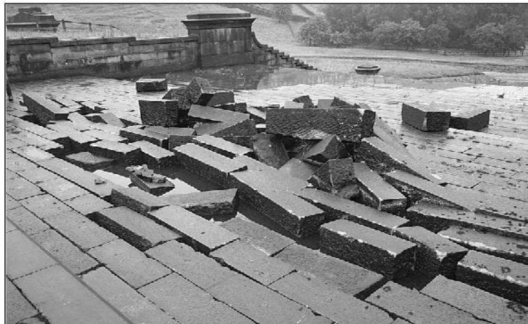
Figure 9. Spillway damage at Butterley IRE
